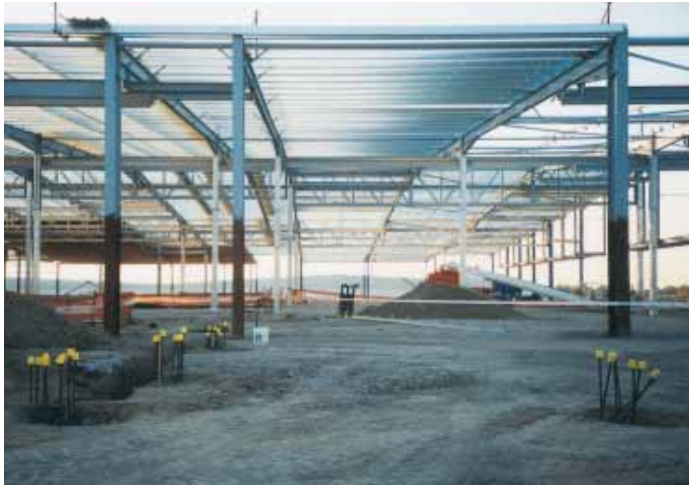
Transfer trusses were used to enable columns to be removed from the typical frame, producing large areas of column-free space.
