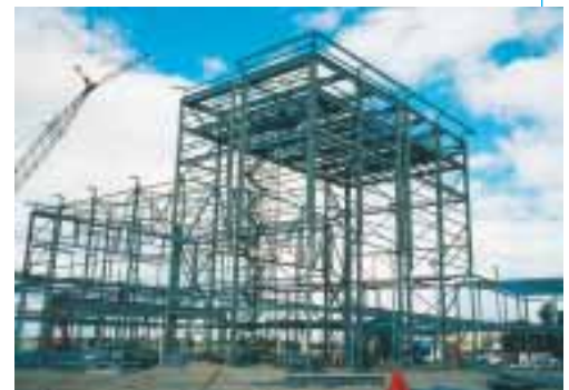
Above, centre: Steel roof trusses, raking members and four leg crucifix frames.
